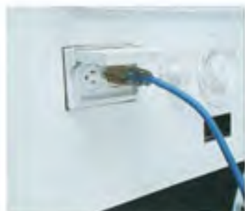
The exterior 120 volt electrical outlet is handy for outside uses.
